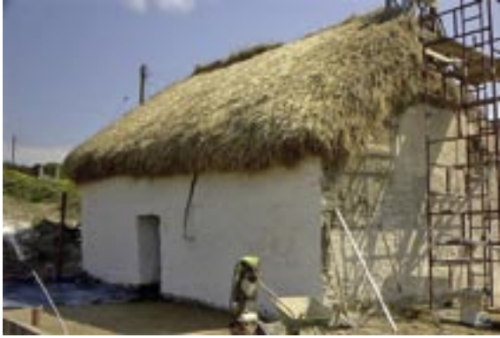
▲ Above the wheatstraw thatch roof Right constructing the chimney cage Uwchben y to gwellt gwenith Dde codi cawell y simnai
